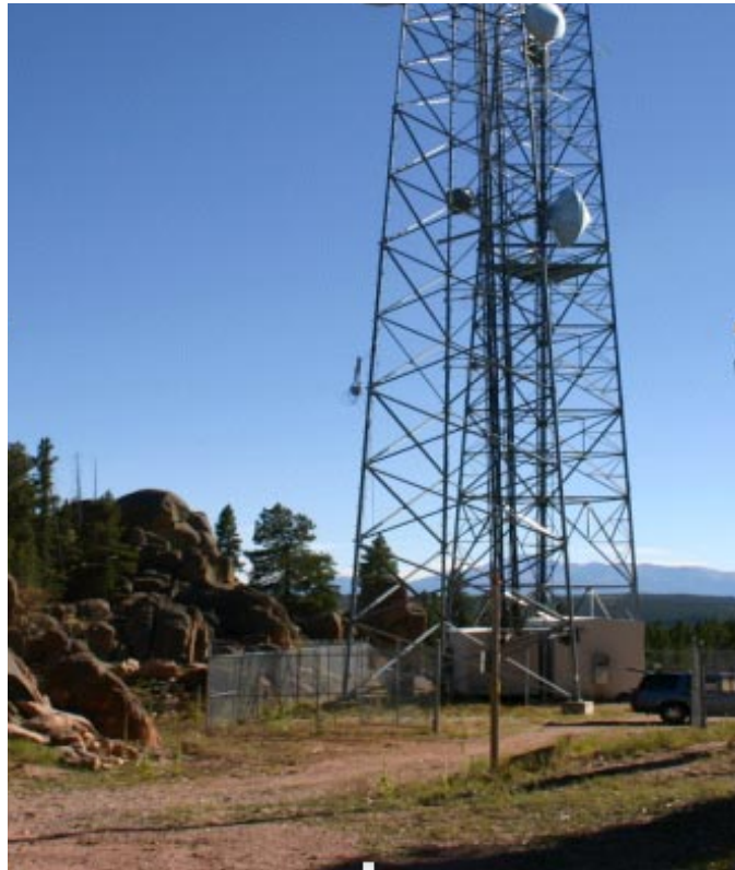
Figure 18 - West Creek Towers (AP Sector Antenna on Left Side at 40' AGL)
